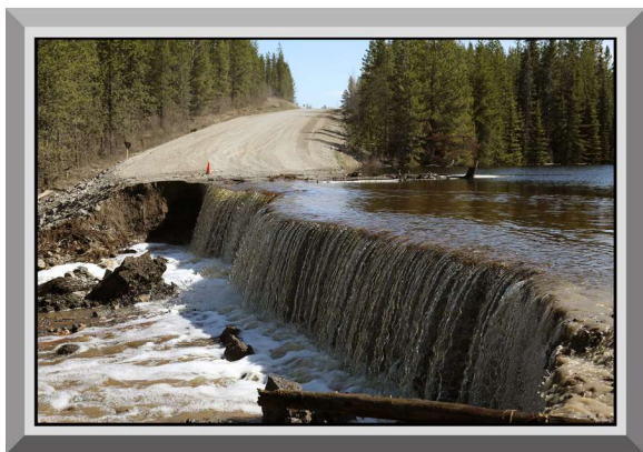
Figure 8.20 Be Wary of Road Washouts.
