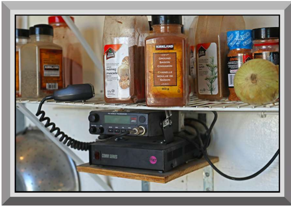
Figure 3.51 VHF Radio in the Kitchen.
